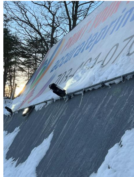
Existing façade sign with LED Up-Lighting
