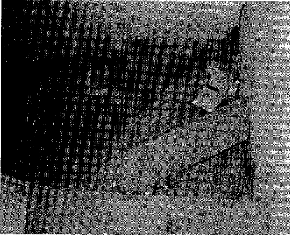
Figure 28: Some of the stair treads, particularly in the winding section, are broken.
