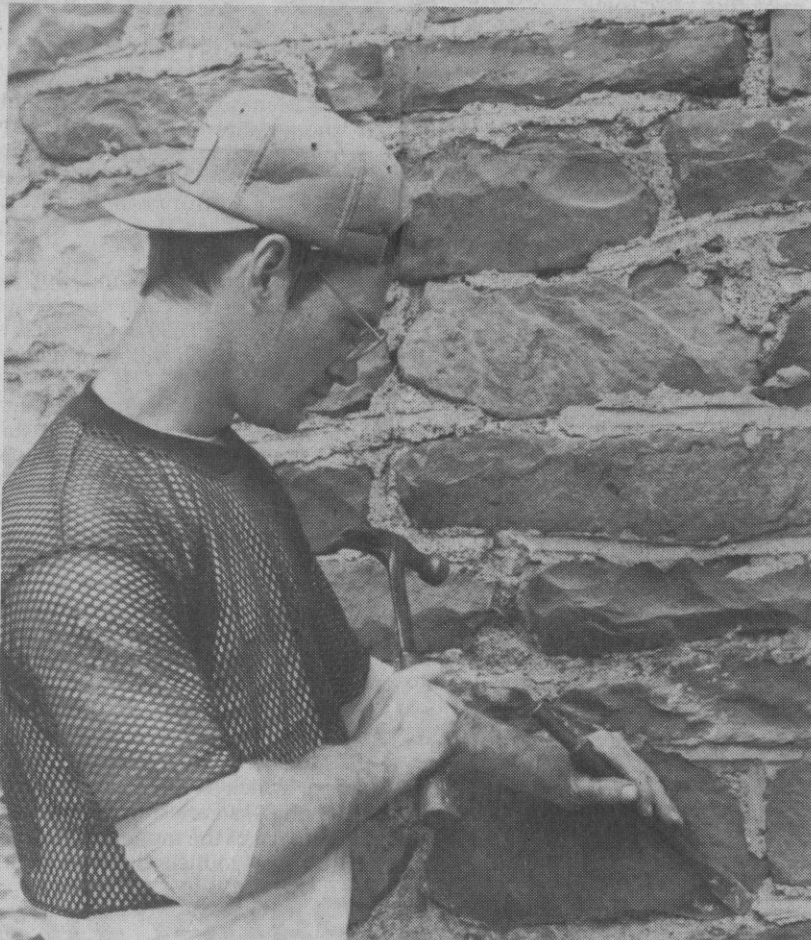
Bennie Scarton Jr. - Journal Messenger Paul Mackert replaces the mortar in one of the walls in one of the outbuildings at the Ben Lomond Manor House property.
