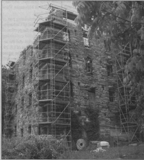
Exterior view of the mill with scaffolding in place for the current Phase II stabilization of the east, north and west walls Harry Leach / the Bull Run Observer
