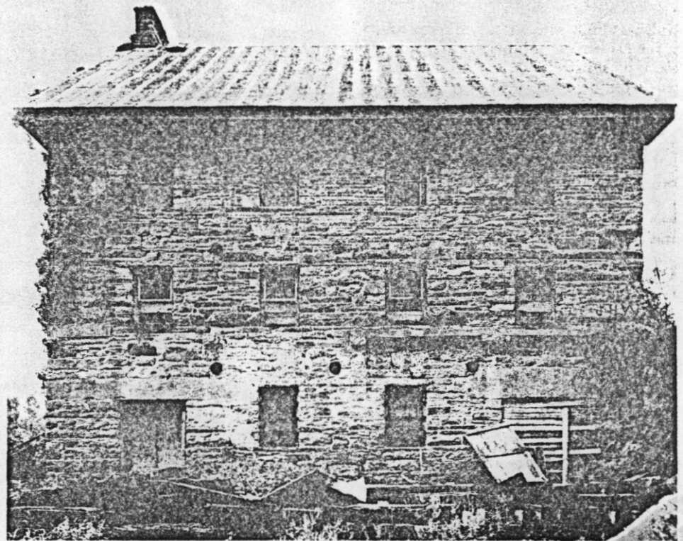
Beverley Mill from the rear (railroad side) as it appears today. The big stone that cracked is over the door at left. The other big one is over the door at right. The crack in the wall zig-zagged its way from top to bottom. (Photo Pioneer America Society/Wm. Edmund Barrett, September, 1971.)
