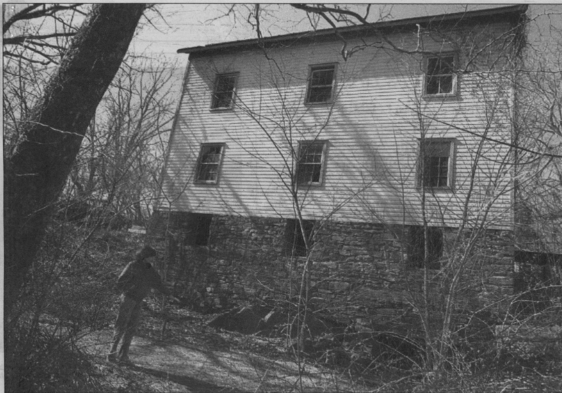
Susan Dudley stands at the base of Buckland Mill, which has been rebuilt several times on the foundation of the original mill. She is concerned that the foundation might suffer permanent damage because of increased water levels and seepage.
