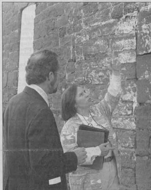
William A. Malcom and Rebecca Stevens get a close up look of the stone work in the Conner House whose construction could date back to the late 1700's.
