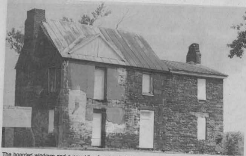
The boarded windows and a crumbling facade of the historic Conner House will be restored to their original conditions.
