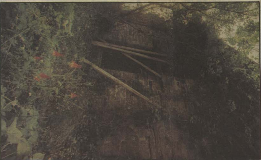
Undergrowth and brush have sprung up around the building with the approach of summer. The mill has been forgotten by all but the history buffs who study Manassas' past.
