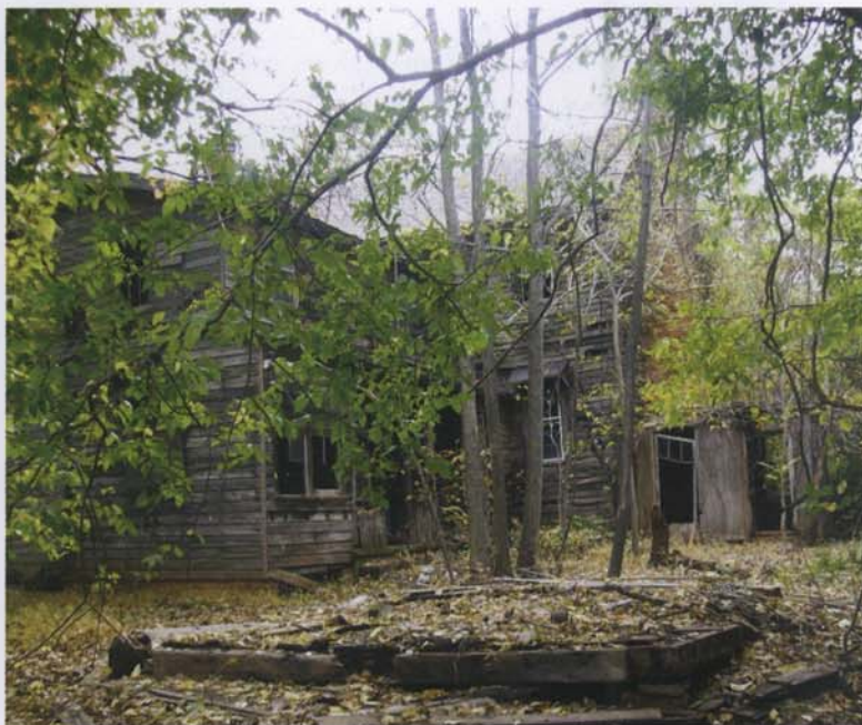
The addition on the rear of the house containing the kitchen and dining room still stands, but is in very poor condition.
