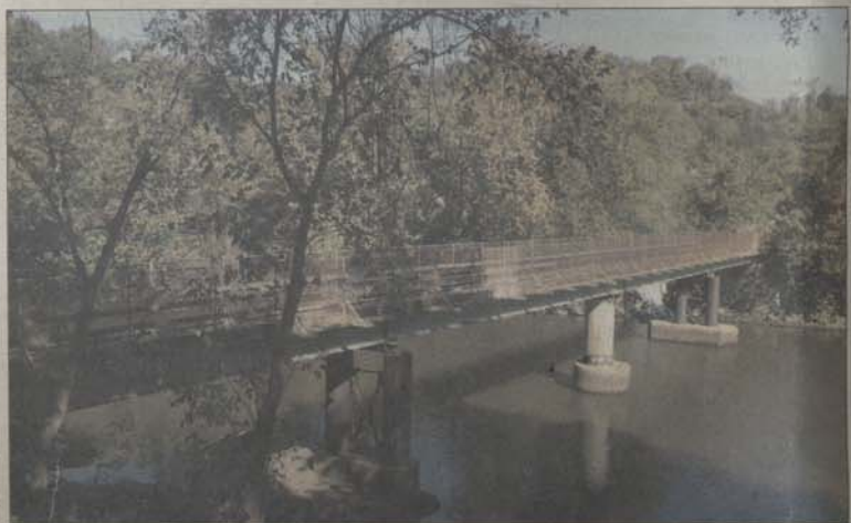
A footbridge now stands at the location of Occoquan's original truss bridge, which was destroyed by flooding caused by Hurricane Agnes in 1972.
