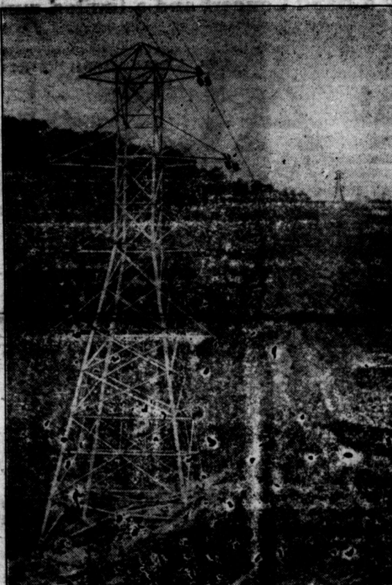
Transmission line between Goshen and Buena Vista. Part of V. P. S. Co.'s interconnected system to give low-cost power throughout its territory.
