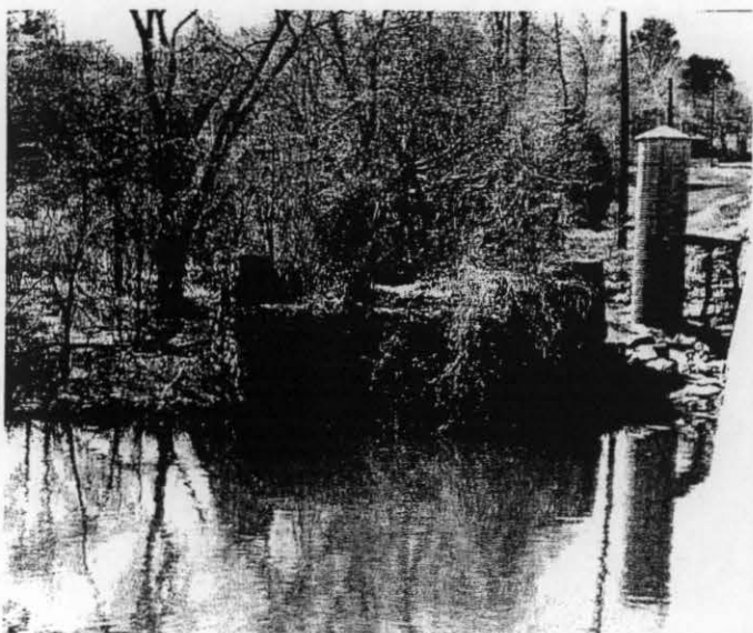
FIGURE 12. Stone bridge abutment at Broad Run, Buckland. This abutment dates to the construction of a timber bridge across Broad Run in 1808, and later served as the support for an iron bridge built in 1890 and replaced in 1927. The road bed of the early turnpike survives for approximately 70 yards to the west of the abutment. Buckland Preservation Society, 2004.
